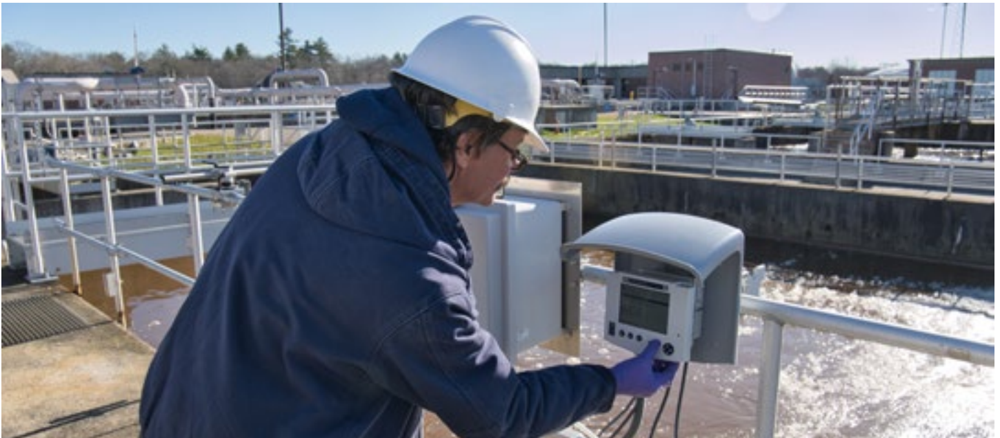
The activated sludge basins are each equipped with a YSI IQ SensorNet system and several sensors to monitor and control their activated sludge process.
